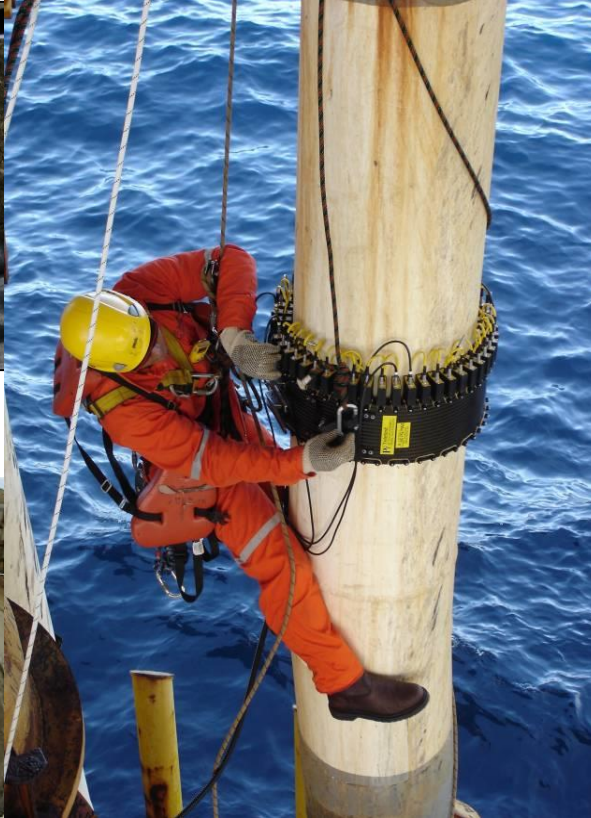
Risers & Topside Pipe-Work
